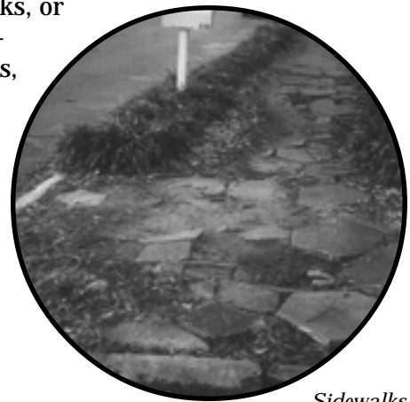
Sidewalks with cracked, uneven pavement and no ramp make it difficult for strollers and wheelchairs to cross.
